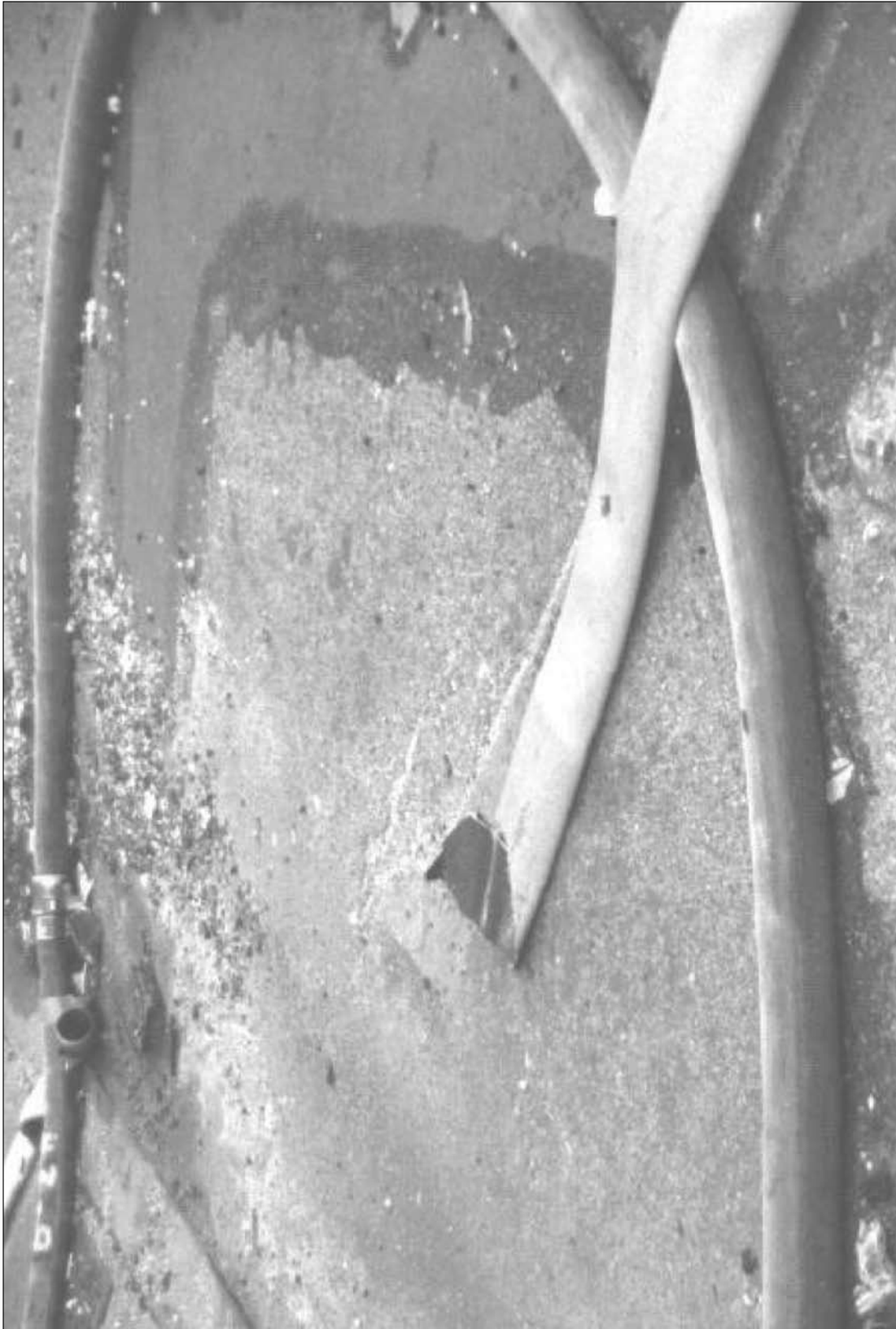
Section of 5-inch hose that was ruptured by falling debris outside the building. Hose lines feeding the standpipes and entering the stairways were damaged several times and had to be replaced at great risk to firefighters. (Shoring boards were later used to protect the hose lines.)
