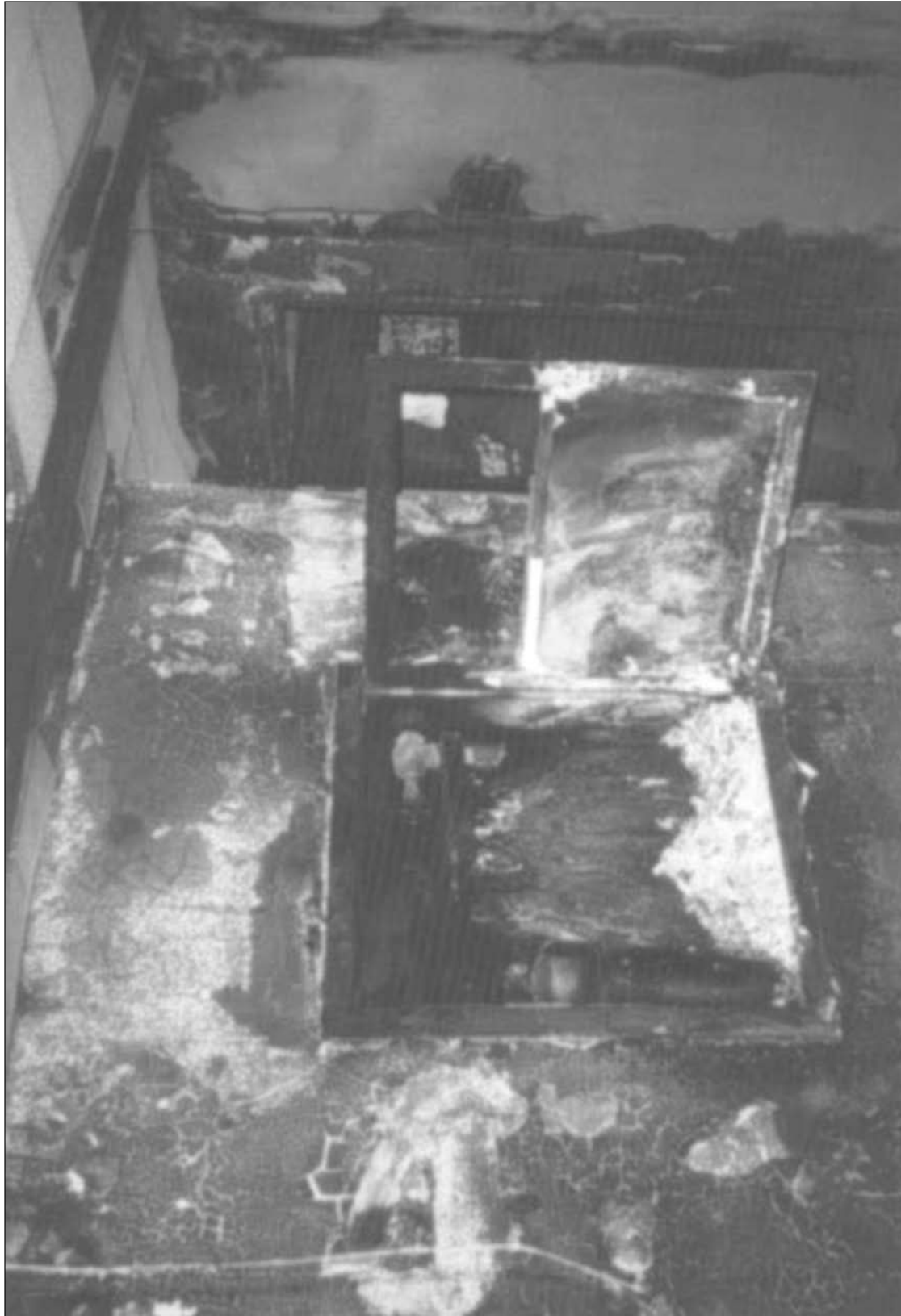
Occupant use standpipe hose cabinet on 26th floor.
