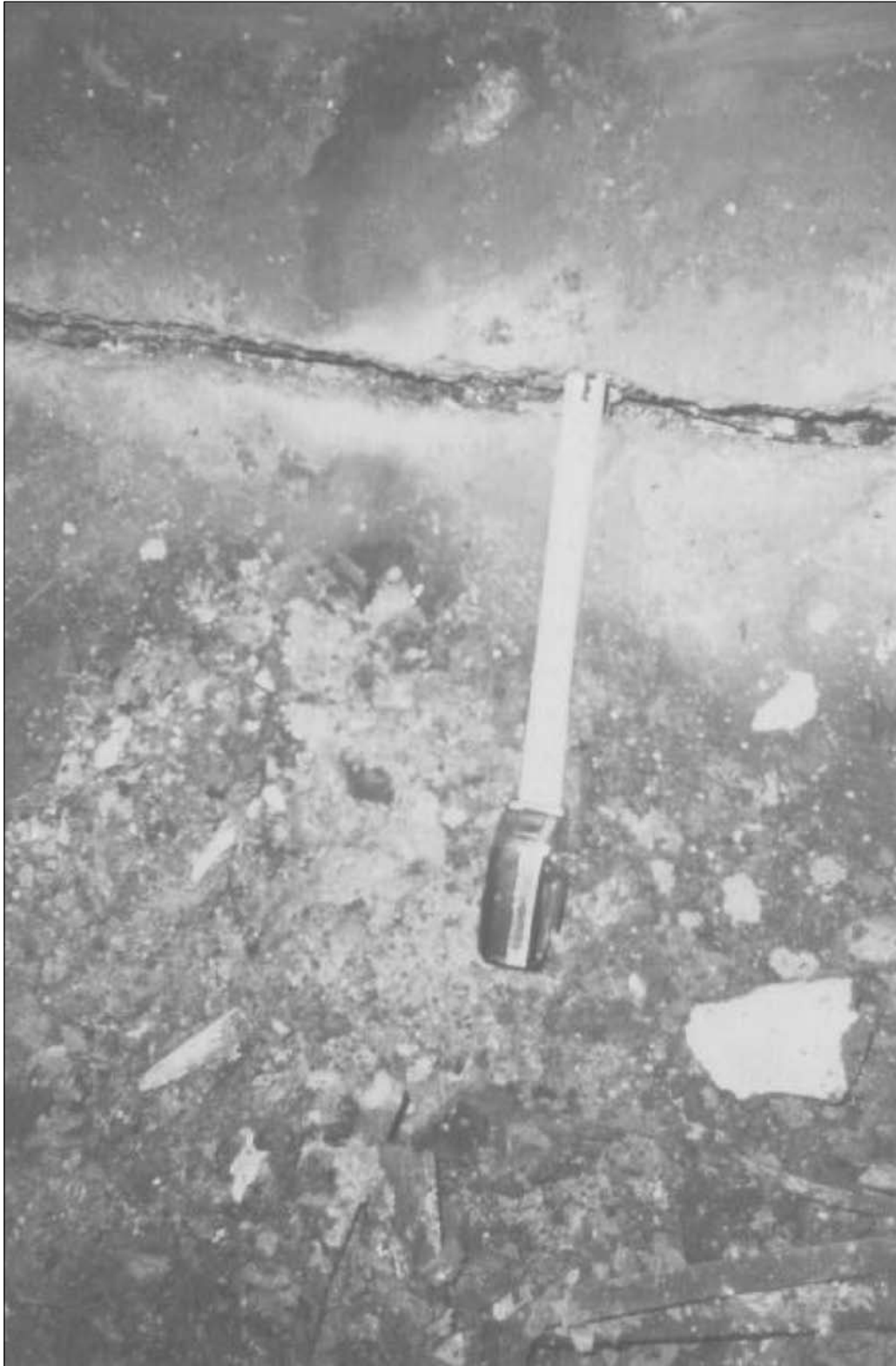
Close-up of crack in concrete floor, 28th floor.
