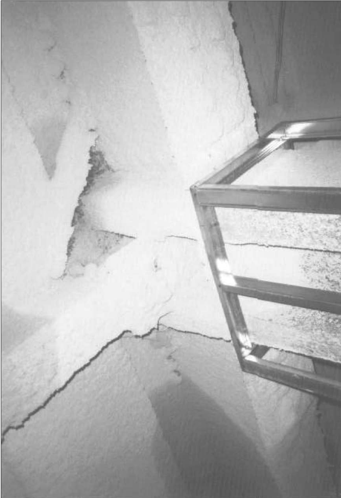
Detail of typical Type 1B construction, 6th floor. Note the spray-applied fireproofing and framing for gypsum wallboard.
