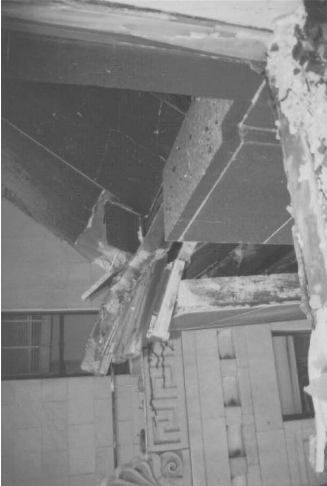
Here and in the next two photos exterior granite panels from the east stair tower were dislodged due to the thermal expansion of the steel frame of the building.
