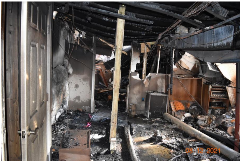
Figure 40: View of basement area, post collapse, where Captain Laird was located and the interior basement wall.
