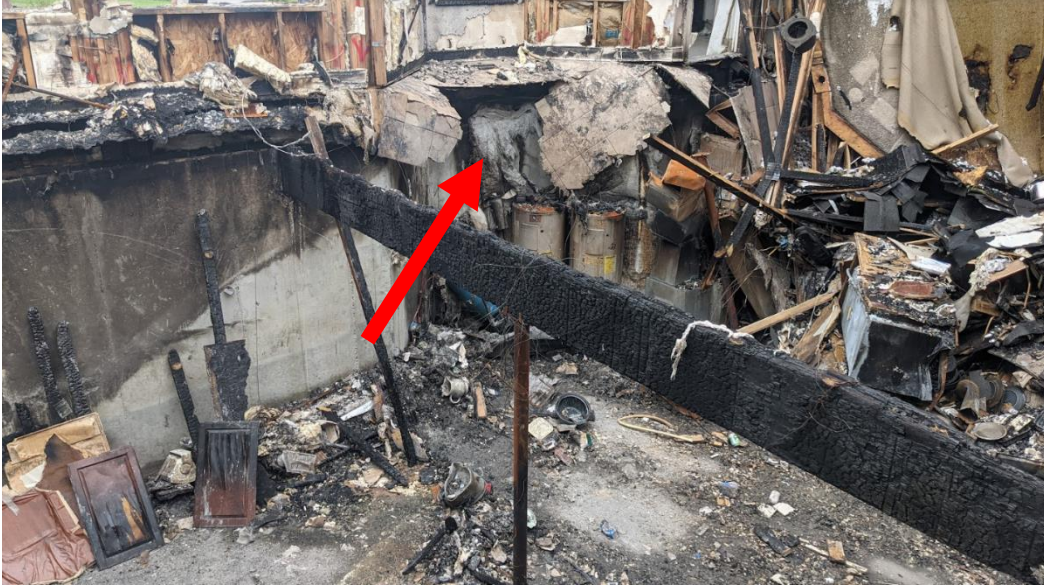
Figure 16: View of basement from Side Bravo. The tile section with the arrow is the area where the collapse occurred sending Captain Laird into the basement.
