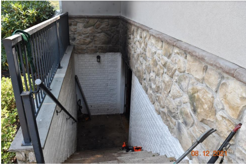
Figure 41: View of the exterior entrance and stairwell on Side Delta of the structure leading into the basement.
