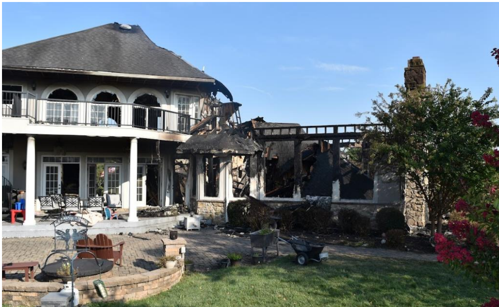
Figure 34: View of Side Charlie of the structure post fire.
